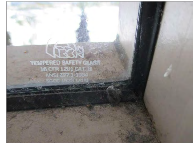
Photo 27: The aluminum framed curtainwall systems in the Atrium area are single pane tempered safety glass manufactured by RC.
