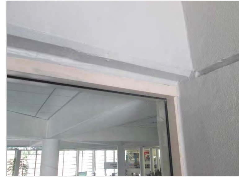
Photo 23: Deteriorated flexible sealant was observed at all exterior perimeters at the frame to wall transitions due to age and exposure to the elements in the Atrium area.
