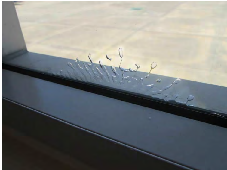
Photo 53: Delamination observed within the single pane tempered safety glass throughout the Concourse area.
