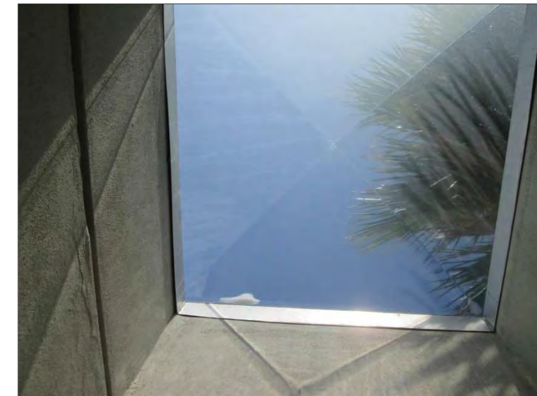
Photo 12: Skylights in the Ticketing area were constructed of a Lexan type plastic material with aluminum framing. The skylight measured approximately 4'7" x 4'7" in size.
