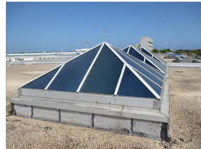
Photo 64: Skylights in the international terminal/baggage claim area. Skylights appeared to be constructed of single pane glass set in structural steel framing. The skylights measured approximately 12' x 13' in size and were in a group of three (totaling 37' x 13').
