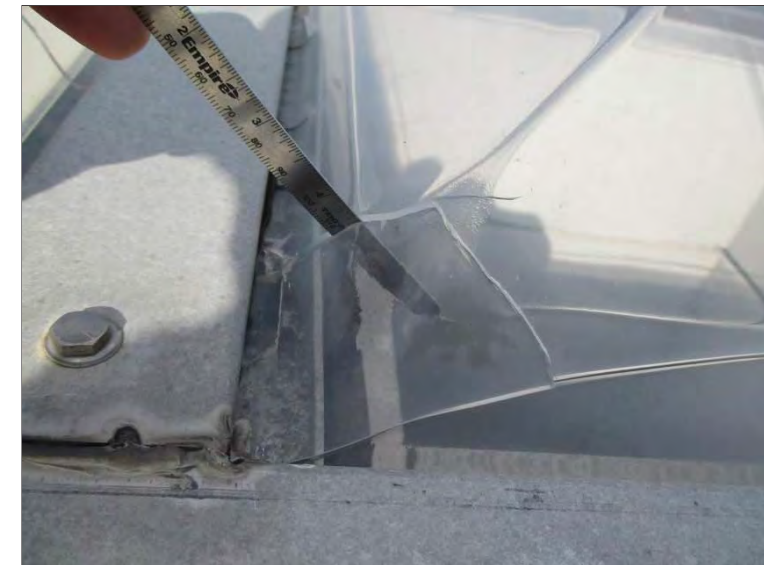
Photo 16: Cracking observed at skylight location in the Ticketing area.
