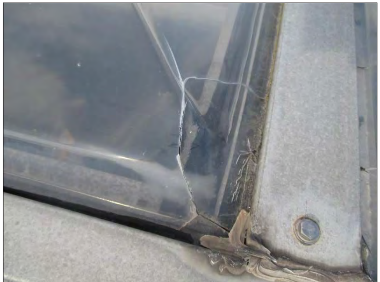
Photo 18: Cracking observed at skylight location in the Ticketing area.
