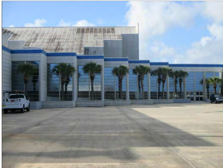
Photo 33: Window assemblies on the north elevation of the Atrium area where PSI performed a visual curtainwall and glazed openings survey to document current condition and note observed deficiencies.
