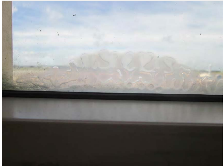
Photo 57: Delamination observed within the single pane tempered safety glass throughout the Concourse area.
