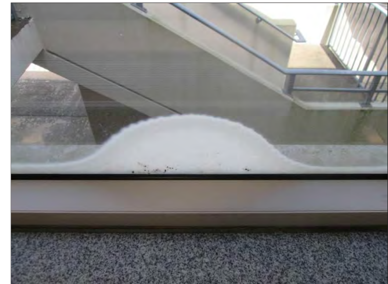
Photo 60: Delamination observed within the single pane tempered safety glass throughout the Concourse area.
