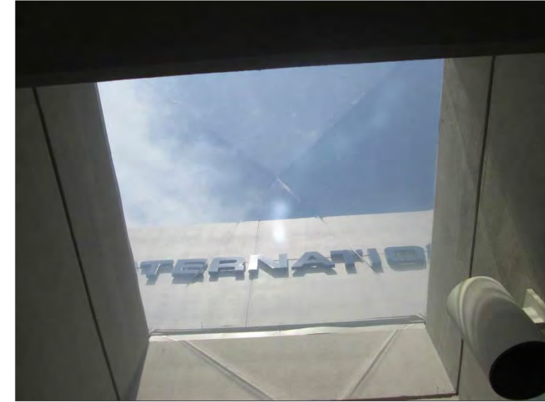
Photo 31: Example of a skylight observed to be in good condition in the Atrium area.
