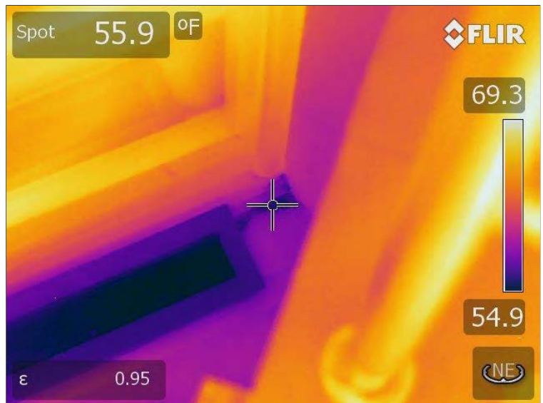
Photo 78: Thermal image of the curtainwall systems on the northwest elevation in the Atrium area where evidence of moisture and water intrusion was observed at the last panel on the right side of the 1 st bay east of the Concourse.
