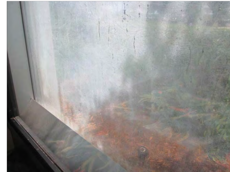
Photo 63: Observed sprinkler head directly outside the window assembly that appears to be directed at the window causing the discoloration.
