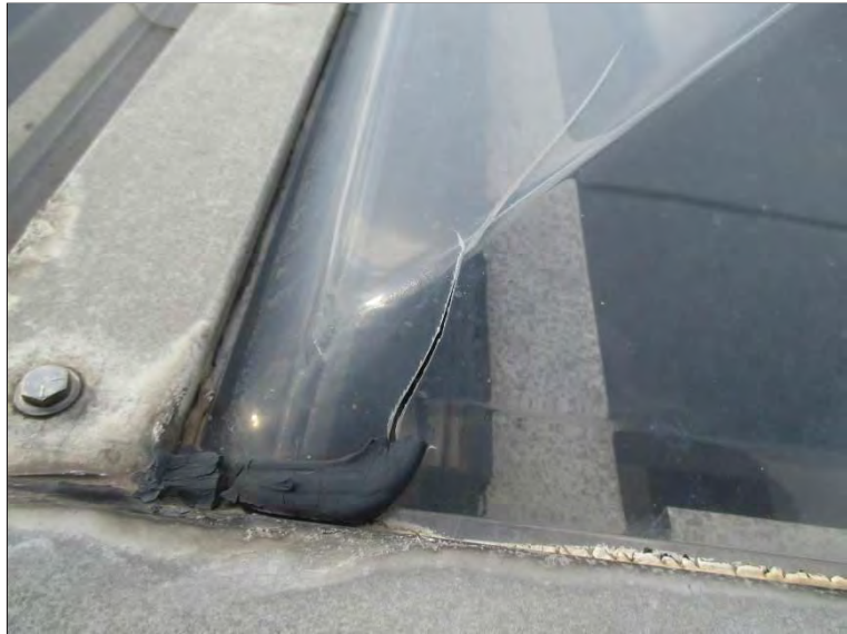
Photo 17: Cracking observed at skylight location in the Ticketing area.
