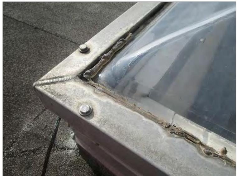
Photo 14: Deteriorated flexible sealant was observed at all perimeter panels to exterior frame transitions due to age and exposure to the elements in the Ticketing area.
