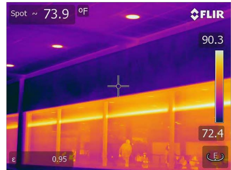
Photo 76: Thermal image of the curtainwall systems throughout the Concourse area. No thermal differences were present indicative of moisture intrusion.
