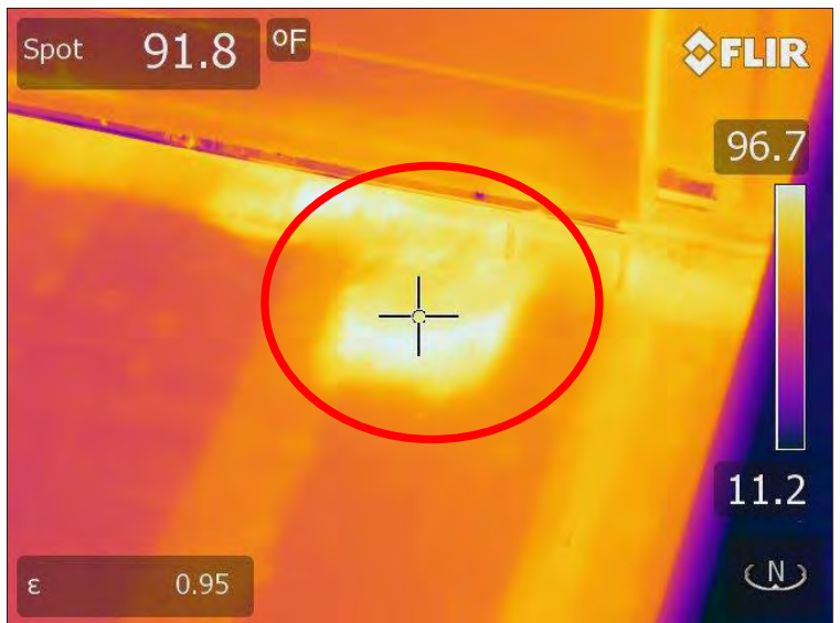
Thermogram 5: Light shaded areas indicate areas of potential trapped moisture under granular capsheet.
