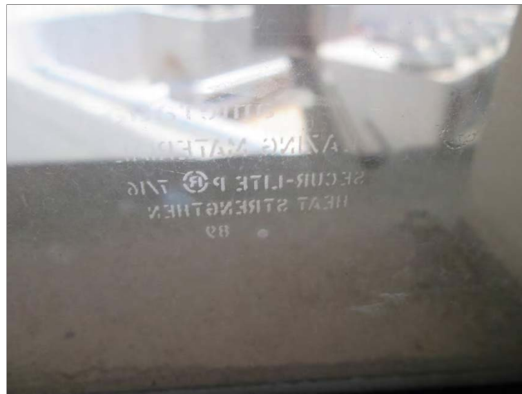
Photo 61: The aluminum framed curtainwall systems are single pane tempered safety glass manufactured by Amerada throughout the Concourse area.
