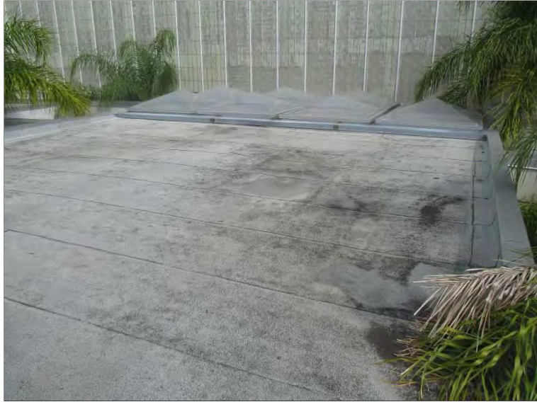
Photo 29: Skylights in the center of the Atrium area where PSI performed visual survey to document current condition and note observed deficiencies.
