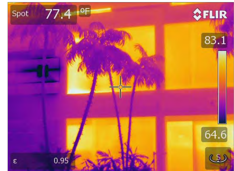
Photo 72: Thermal image of the curtainwall systems on the south elevation of the Atrium area. No thermal differences were present indicative of moisture intrusion.
