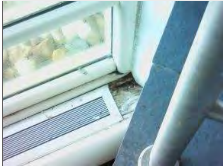
Photo 77: Digital image of the curtainwall systems on the northwest elevation in the Atrium area where evidence of moisture and water intrusion was observed at the last panel on the right side of the 1 st bay east of the Concourse.
