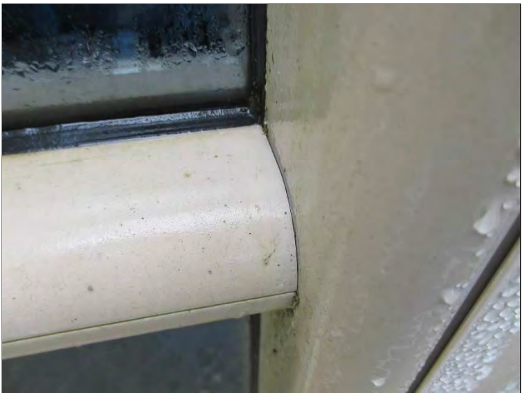
Photo 44: Missing flexible sealant on the exterior of the rounded aluminum framing applied to at the horizontal to vertical transitions in the Atrium area.
