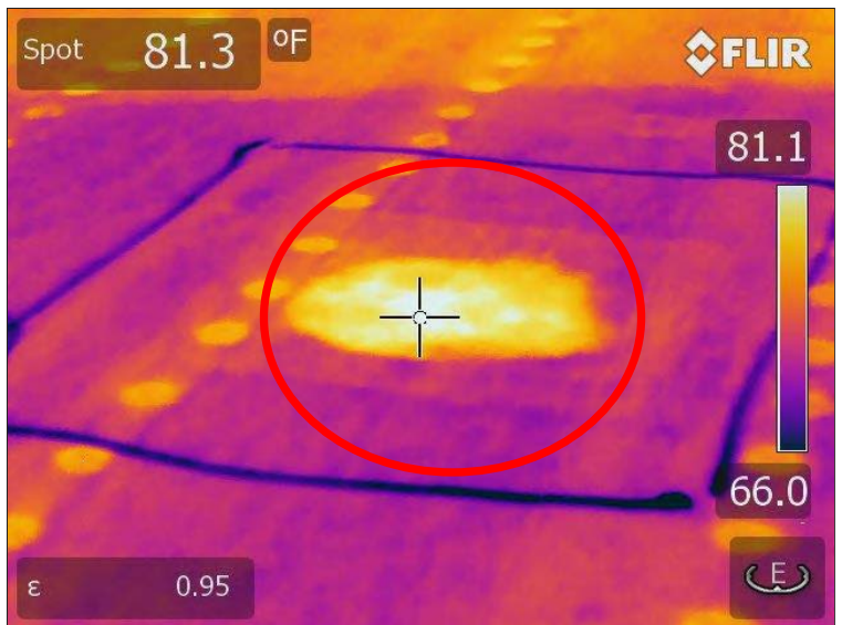
Thermogram 15: Light shaded areas indicate areas of potential trapped moisture under granular capsheet.
