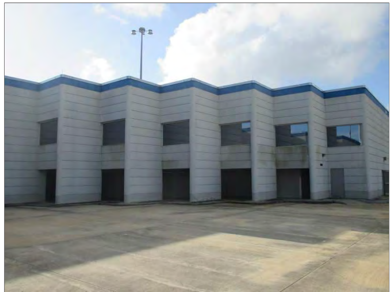
Photo 50: Window assemblies in the Concourse area throughout the west elevation where PSI performed a visual curtainwall and glazed openings survey to document current condition and note observed deficiencies.
