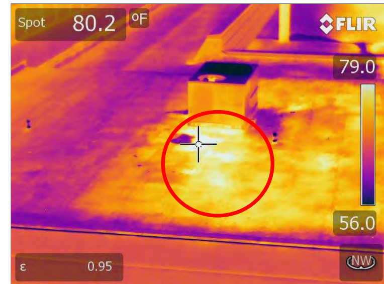
Thermogram 8: Light shaded areas indicate areas of potential trapped moisture under granular capsheet.
