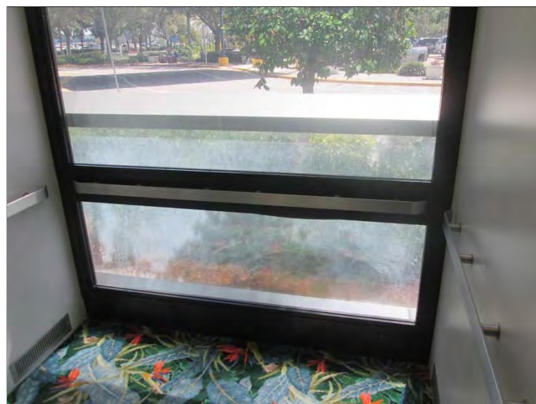
Photo 62: Discolored bottom lite associated with the elevator in the baggage claim area. The window currently appears to be functioning as designed and is only aesthetically unappealing.
