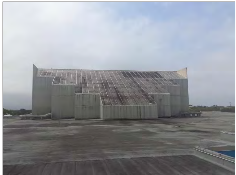
Photo 22: Overview of translucent panels on south elevation of elevated structure on Atrium roof.
