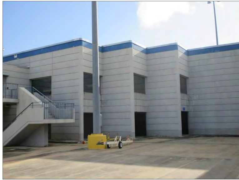
Photo 49: Window assemblies in the Concourse area throughout the west elevation where PSI performed a visual curtainwall and glazed openings survey to document current condition and note observed deficiencies.
