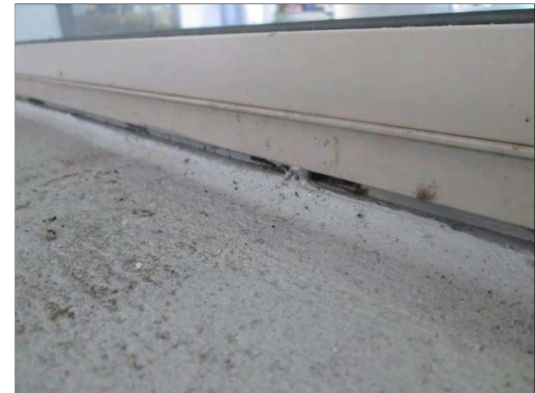
Photo 24: Deteriorated flexible sealant was observed at all exterior perimeters at the frame to wall transitions due to age and exposure to the elements in the Atrium area.
