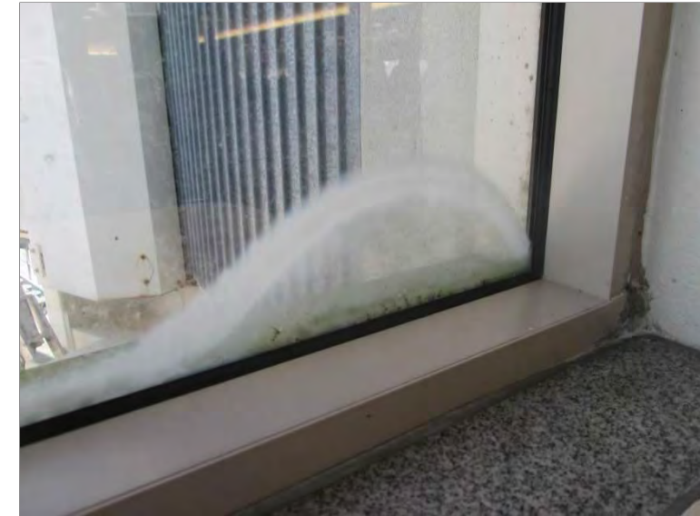
Photo 59: Delamination observed within the single pane tempered safety glass throughout the Concourse area.
