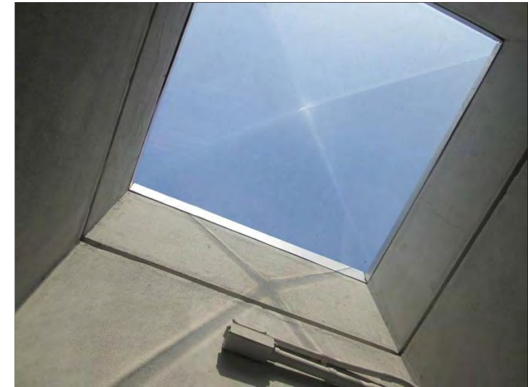
Photo 32: Example of a skylight observed to be in good condition in the Atrium area.
