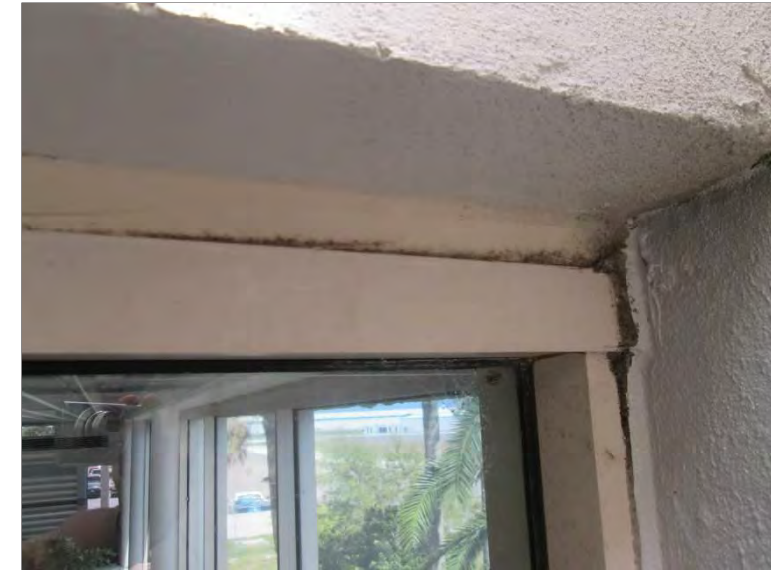
Photo 3: Deteriorated flexible sealant was observed at all exterior perimeters at the frame to wall transitions due to age and exposure to the elements.
