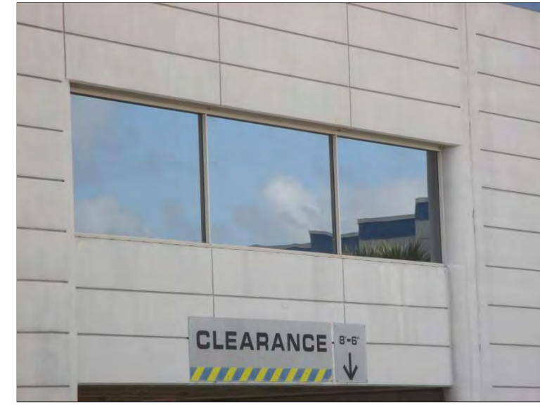
Photo 51: Window assemblies in the Concourse area throughout the west elevation where PSI performed a visual curtainwall and glazed openings survey to document current condition and note observed deficiencies.
