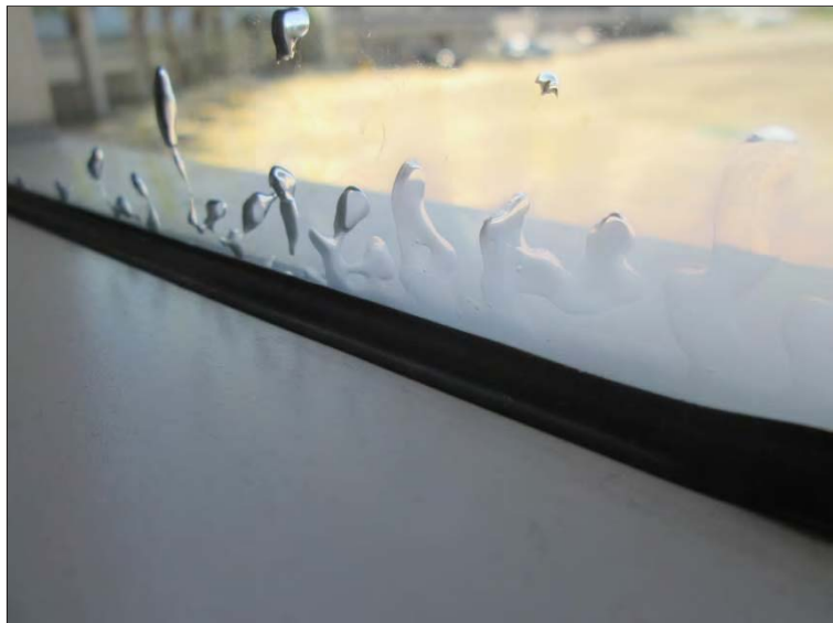
Photo 54: Delamination observed within the single pane tempered safety glass throughout the Concourse area.
