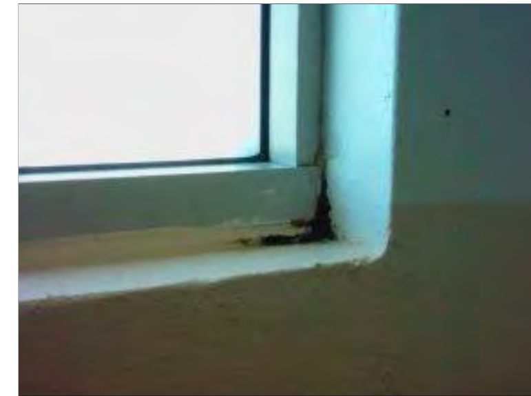
Photo 79: Digital image of the curtainwall systems on the west elevation in the Concourse area where evidence of moisture and water intrusion was observed at the set of three aluminum framed curtainwall systems leading to the Atrium at the lower right corner of the north panel at the frame to interior gypsum wallboard transition.
