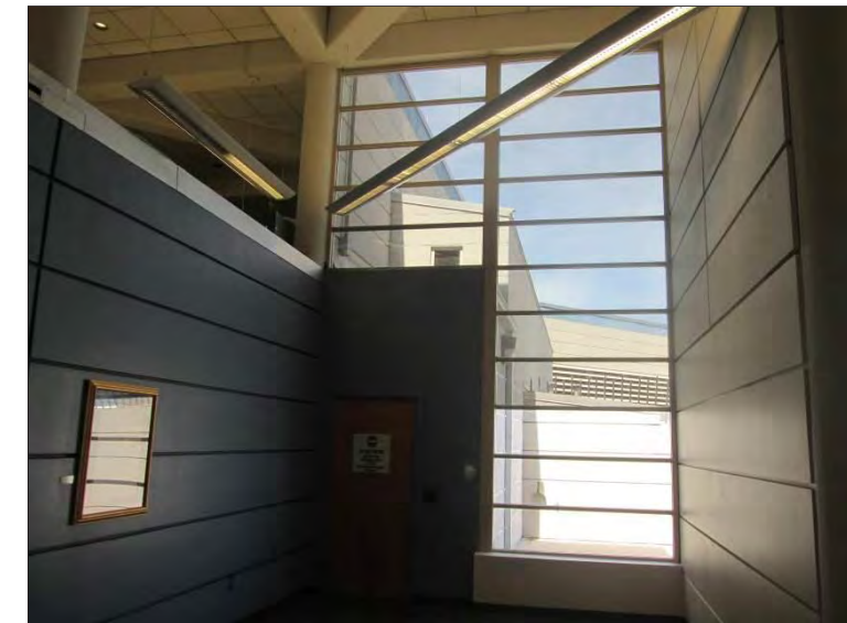
Photo 36: Interior view of window assemblies on the northeast elevation of the Atrium area where PSI performed a visual curtainwall and glazed openings survey to document current condition and note observed deficiencies.
