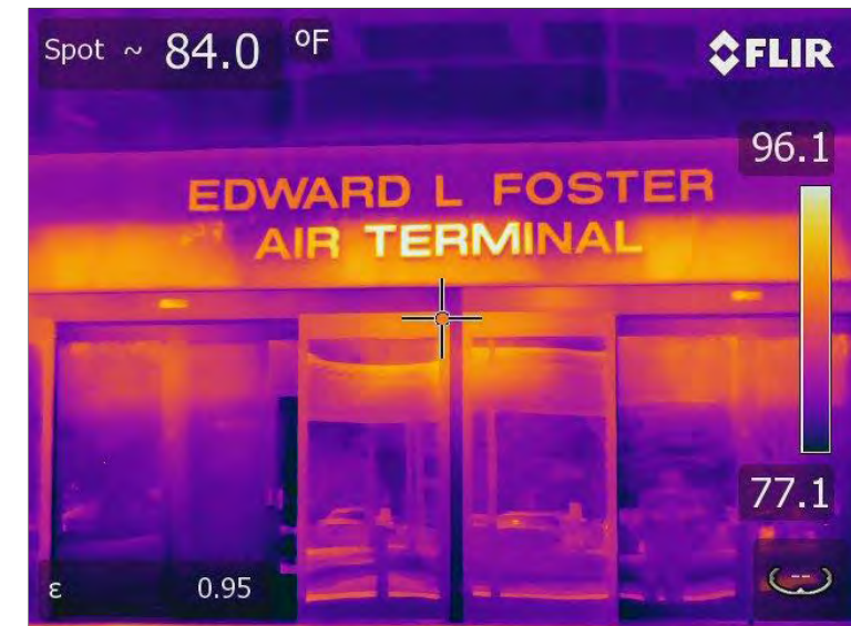
Photo 68: Thermal image of the main entrances to the Atrium area. No thermal differences were present indicative of moisture intrusion.
