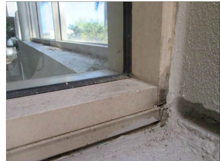
Photo 4: Deteriorated flexible sealant was observed at all exterior perimeters at the frame to wall transitions due to age and exposure to the elements.
