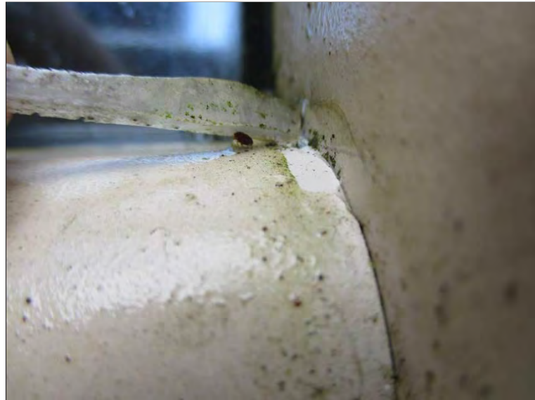
Photo 45: Deteriorated or pulling away flexible sealant on the exterior of the rounded aluminum framing applied to at the horizontal to vertical transitions in the Atrium area.
