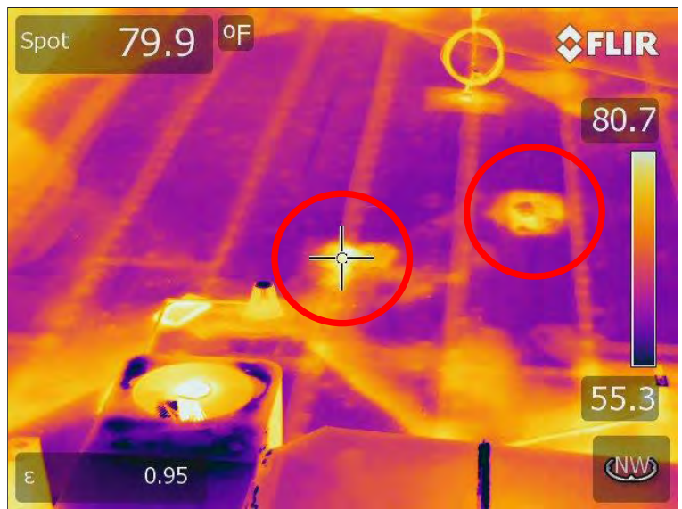
Thermogram 1: Light shaded areas indicate areas of potential trapped moisture under granular capsheet.
