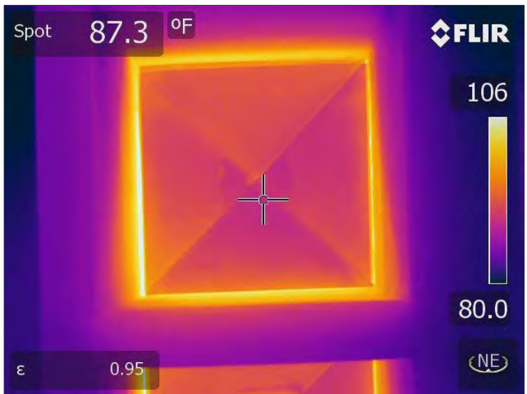
Photo 74: Thermal image of the skylights associated with the Ticketing area. No thermal differences were present indicative of moisture intrusion.
