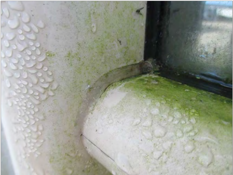
Photo 43: Flexible sealant on the exterior of the rounded aluminum framing applied to at the horizontal to vertical transitions in the Atrium area.
